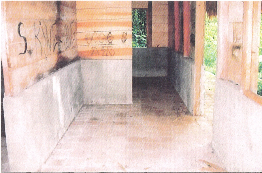
5. Inside view of cabana grande, most wood and tile in good shape. Notice the good condition of the blonde “hormigo” wood compared to the darker “palo de sangre” wood on the left side of picture.
